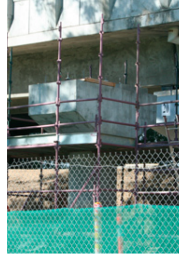
Images on this page show construction progress and the noisewall soon to be replaced by a temporary barrier.
