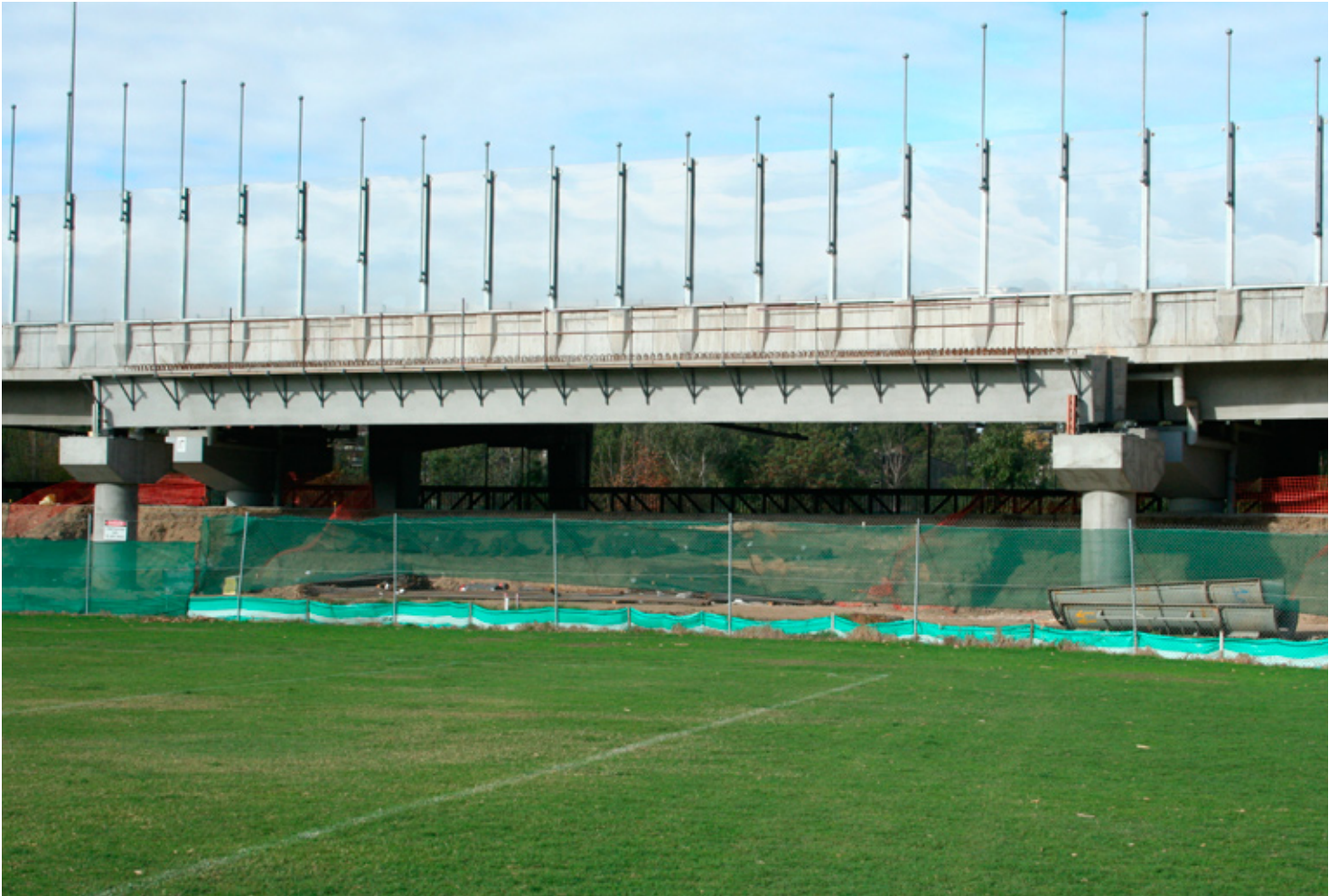
New concrete supports and a recently-installed concrete beam for the widened tollway provide a changing backdrop for the Melville Oval.
