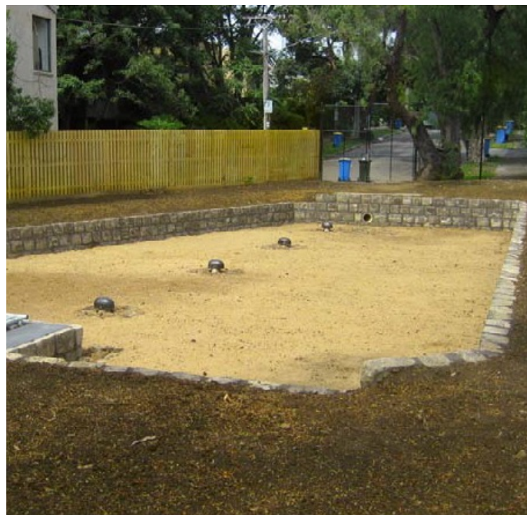
TOP: THE HAMBLEDON ROAD RAIN GARDEN AS IT NOW APPEARS BOTTOM: THE RAIN GARDEN UNDER CONSTRUCTION IN 2011
