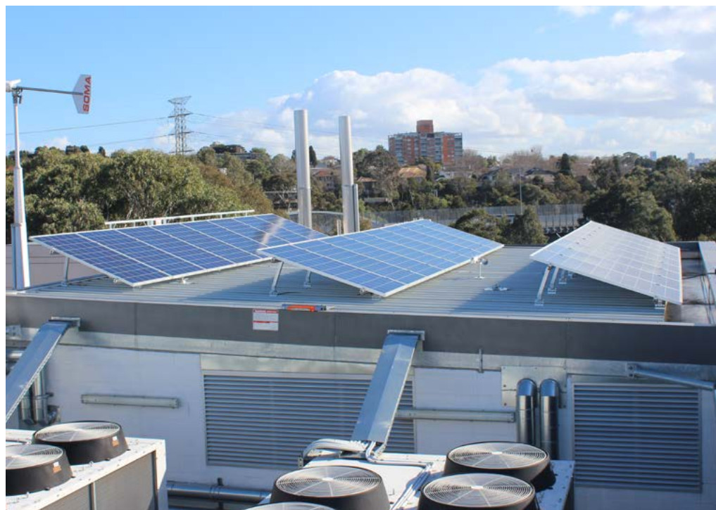
TOP: PHOTOVOLTAIC PANELS ON THE CENTRE FOR SCIENCE ROOF BOTTOM: SOLAR PANELS FACING MORRISON STREET
