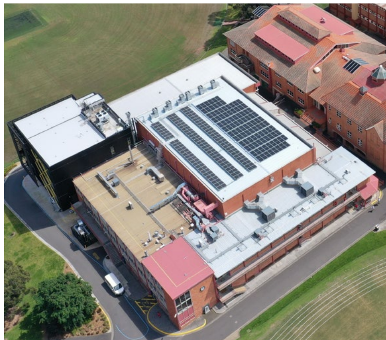
ABOVE: SOLAR PANELS ON THE GLENN CENTRE ROOF. BELOW: THE SOLAR PANEL INSTALLATION COVERS THE UPPER GYM ROOF OF THE GLENN CENTRE
