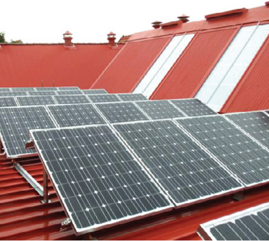
First solar steps – some of the panels recently installed on Scotch College roofs
