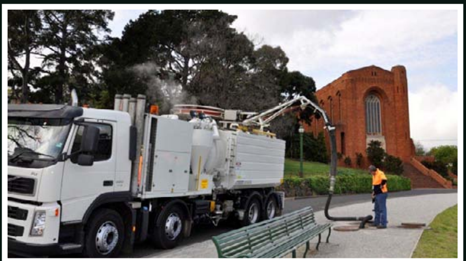
A gross pollutant trap on the eastern side of the Main Oval being cleaned by a contractor.
